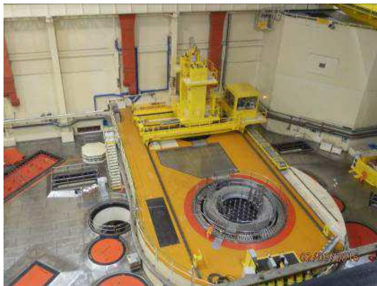
Figure 1: SF pool and transfer cask shaft during reactor refuelling
