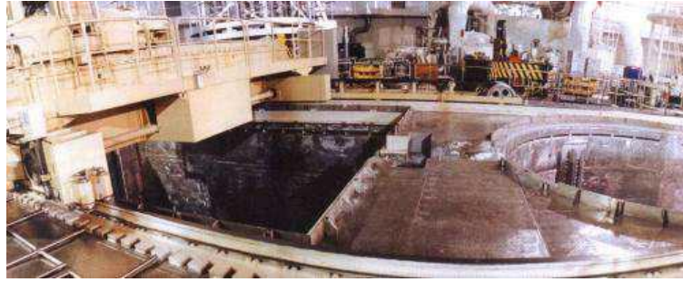
Figure 3: Uncovered SF pool at NPP Temelin
